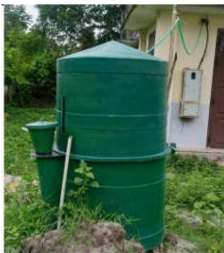
Biogas Plant I
