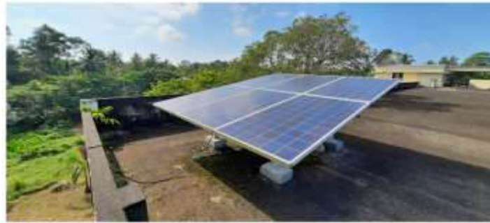
Solar Power Plant
