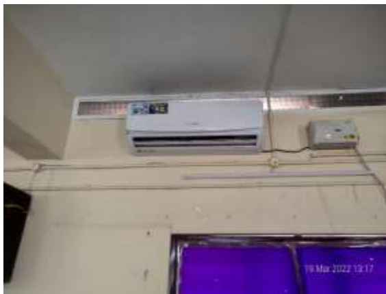
Image 3.d : Energy efficient air conditioner in Seminar Hall
